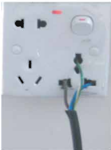
Faulty electric connection
