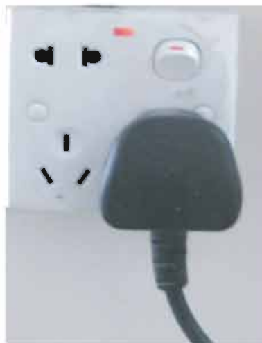
Proper electric connection
