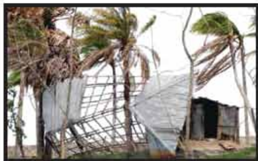
The wind is blowing the roof away.
